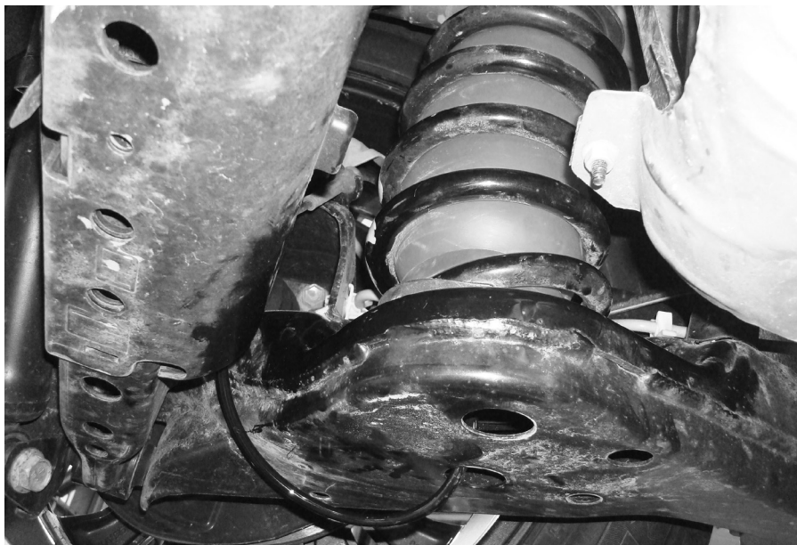
Inside, forward of axle view of driver's (left) side installation
