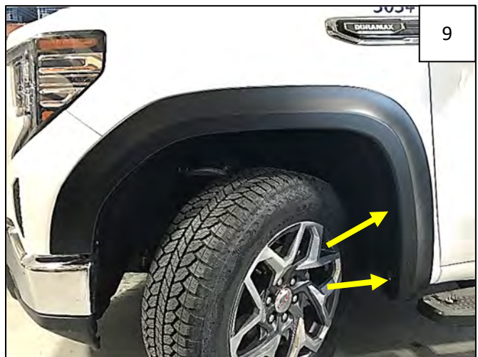
9 Install 2 factory T-15 Tox screws through rearward holes in flare and into factory holes in fender.
