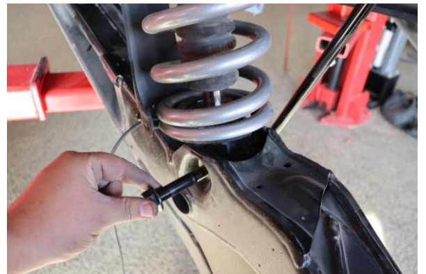
Step 24. Install lower shock mount nut and bolt. Tighten to manufacturer specification using 2 21mm sockets.
